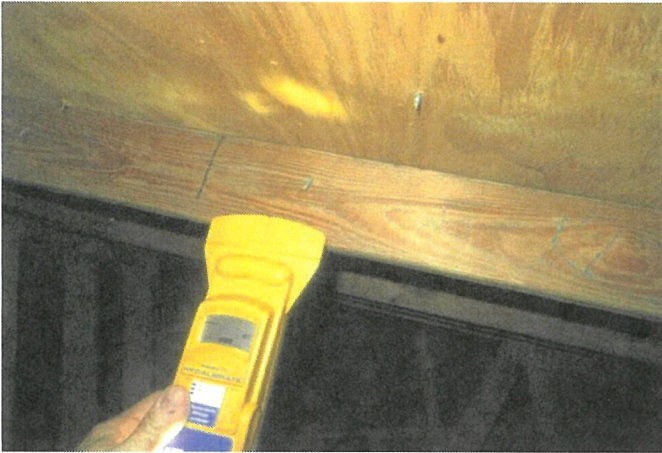
Nail location verified
